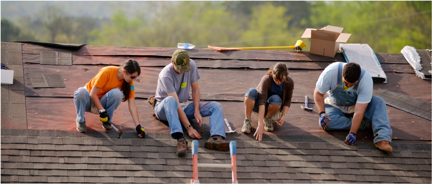
Fahe Member Knox County Habitat for Humanity hosted a Blitz Build where homeowners and the community came together to build 6 homes in 7 days.
