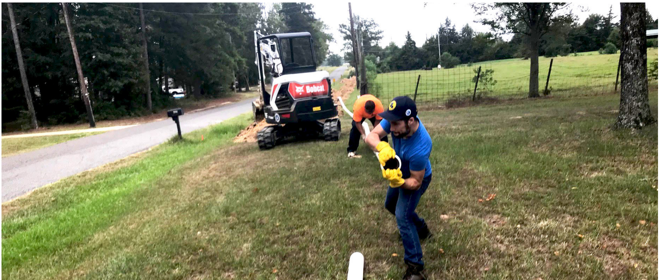
Communities Unlimited supports infrastructure projects like this line extension in the field.
